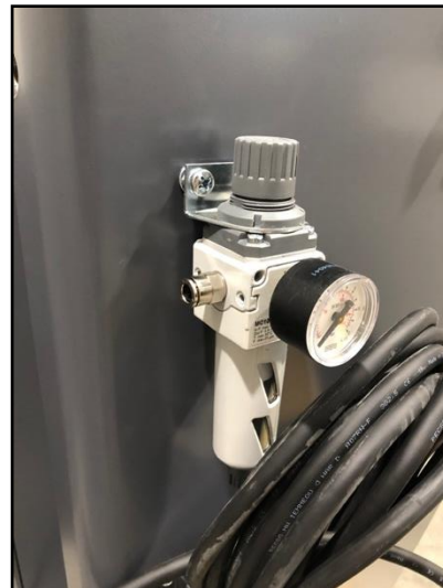
Fig.9 Filter with pressure gauge
